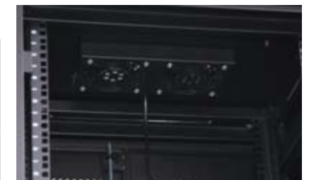
Fan units for dissipate heat
