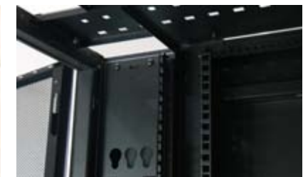
Cable management rails in rear
