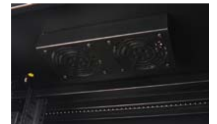
Fan units for dissipate heat
