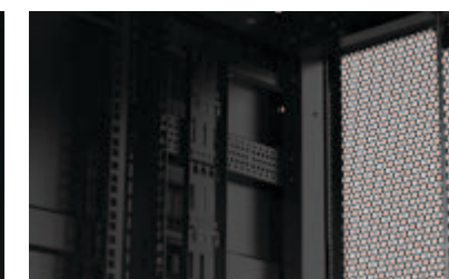
Cable management rails in rear
