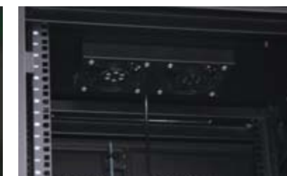
Fan units for dissipate heat
